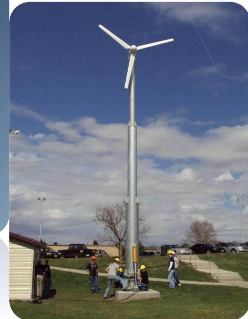
3 Kilowatt Southwest Turbine
