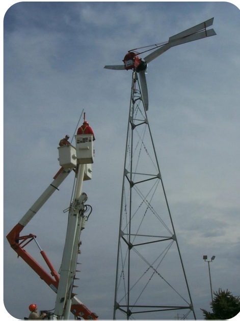
10 Kilowatt American Energy
