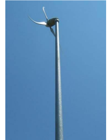
2.4 kW Skystream Turbine at UNL
